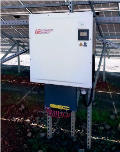
In terms of post-installation monitoring and maintenance, many EPCs prefer string inverters.
